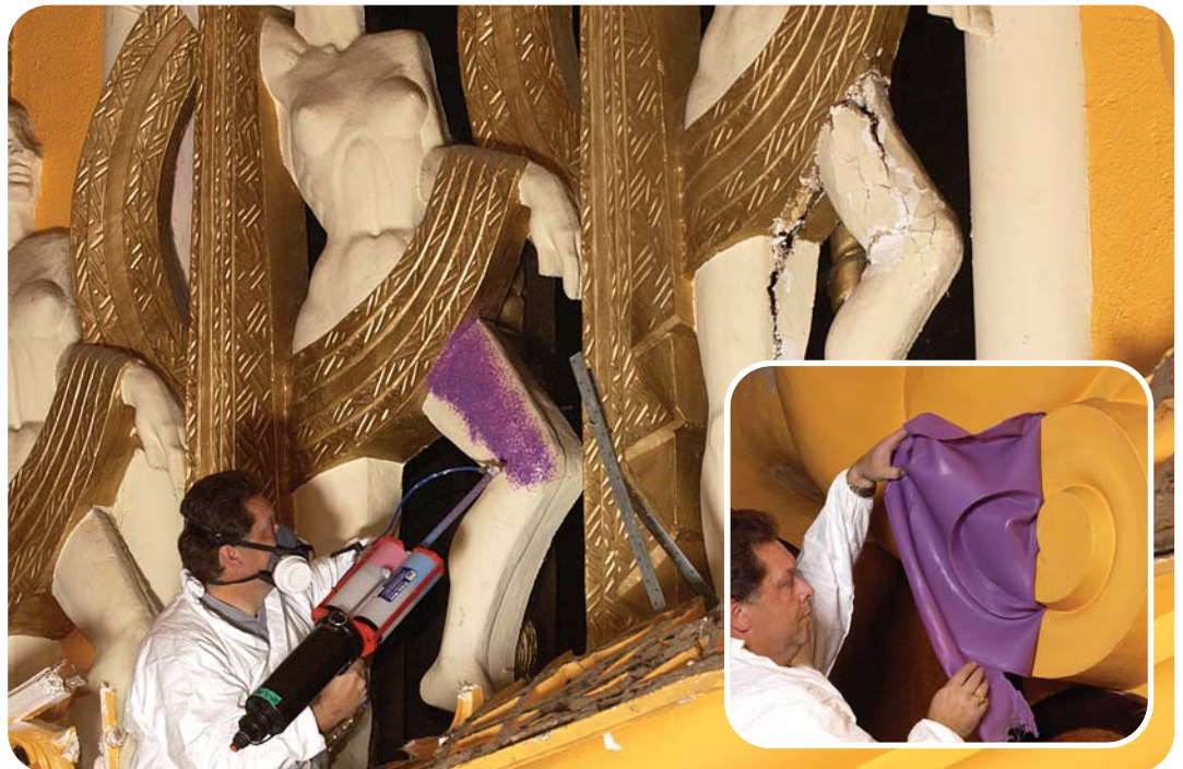
The EZ-Spray System spraying Silicone Rubber for detailed restoration work in a Grade 2 listed building
